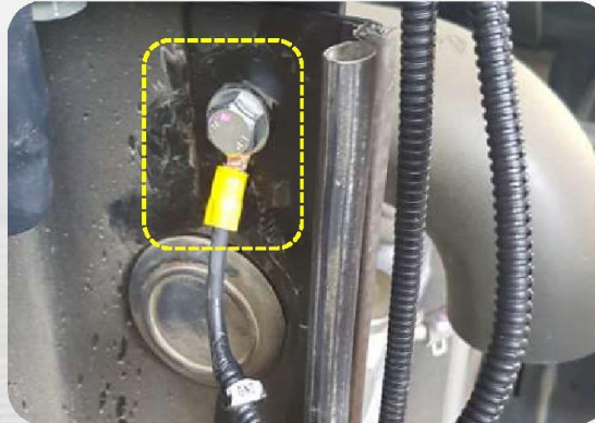
GND connection(equipment frame)
