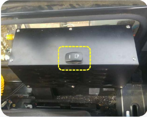
Switch(embedded in the air compressor)
